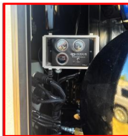
Air Excavation Controls
