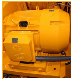
40 HP Electric Motor
