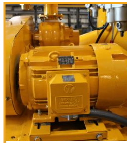
30 HP Electric Motor
